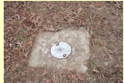
The wells being installed will be flush-mounted and will look similar to the picture above.
